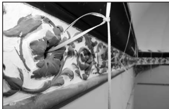
The sockets in the flower frieze are being prepared for new wiring
